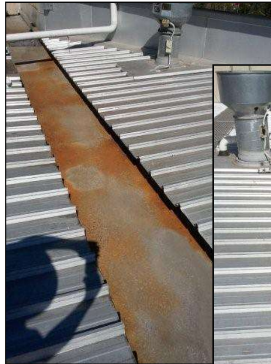
Rusted box gutter corroding and leaking
